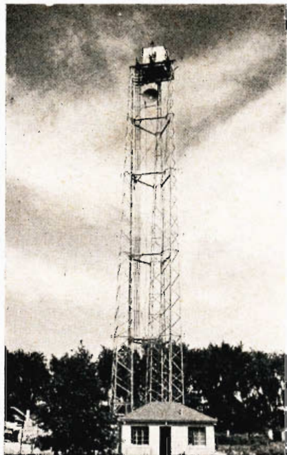
Relay equipment towers at Michigan City, Ind. A 6 foot parabolic reflector is seen being hoisted to its location on west wall of penthouse.
